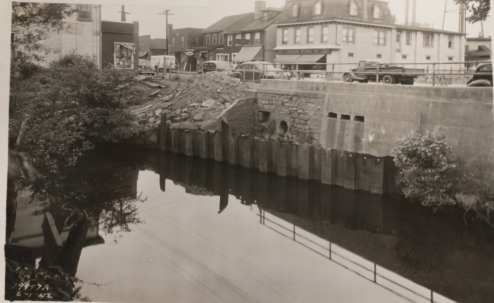
Flood Protection Works at Mt. Holly, N. J. Contract No. W-697-eng-3460. Contractor: Foundations & Excavations, Inc. 1997 - Temporary cofferdam at south end of by-pass channel - camera on Mt. Holly Textile Co. bridge, facing northwest.
