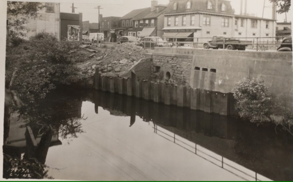
Flood Protection Works at Mt. Holly, N. J. Contract No. W-697-eng-3460. Contractor: Foundations & Excavations, Inc. 1937 - Temporary cofferdam at south end of by-pass channel - camera on Mt. Holly Textile Co. bridge, facing northwest.
