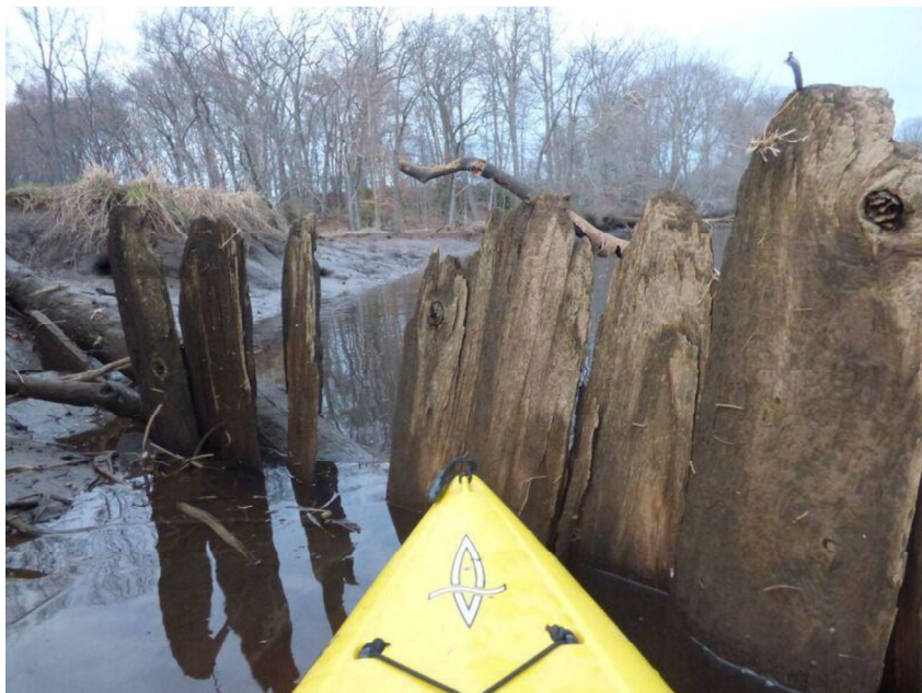
Figure 19 Skeletal remains of Bulkhead and loading dock protruding from creek at low water.
